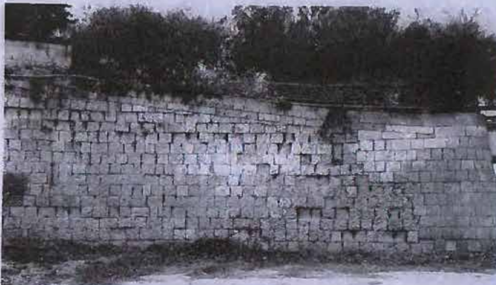
Counterscarp facing south-east showing further surface erosion.
