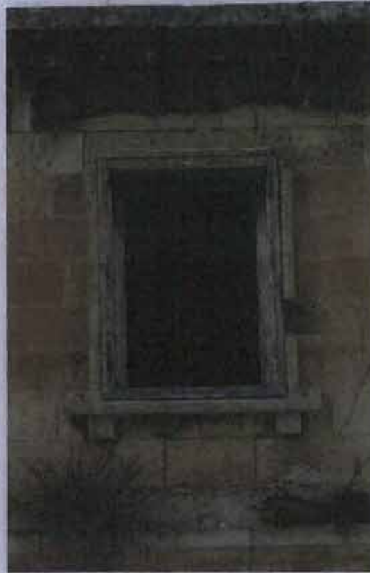
Figure 10: Photo showing bad detailing of timber frame
