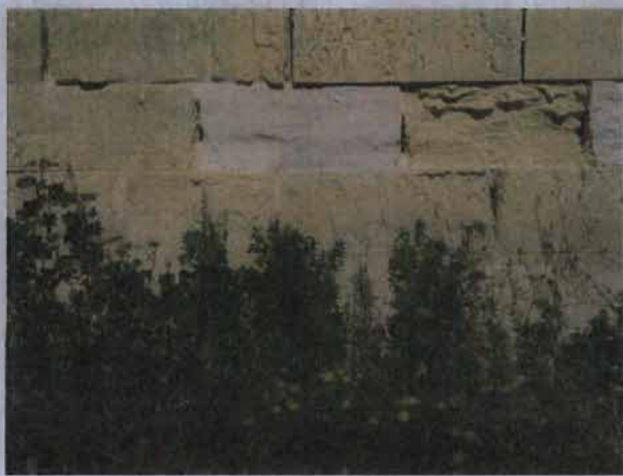
The historic stables – vegetation and surface erosion.
