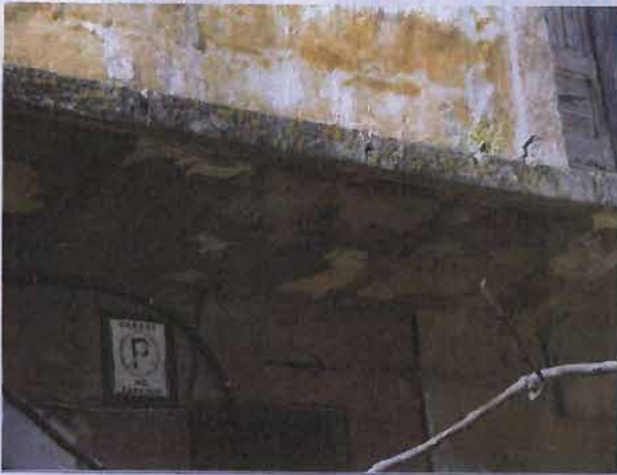
The historic stables – accretions, discoloration and the bad existing condition of the balcony.
