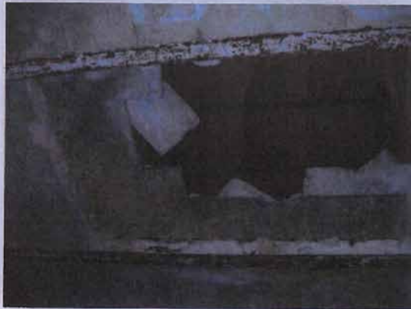
Figure 3: Photos taken from ground floor showing the bad state of the ceilings
