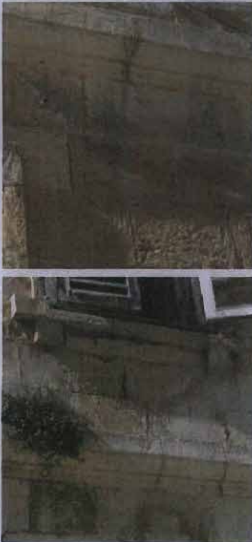
The historic stables – efflorescence and differential erosion.
