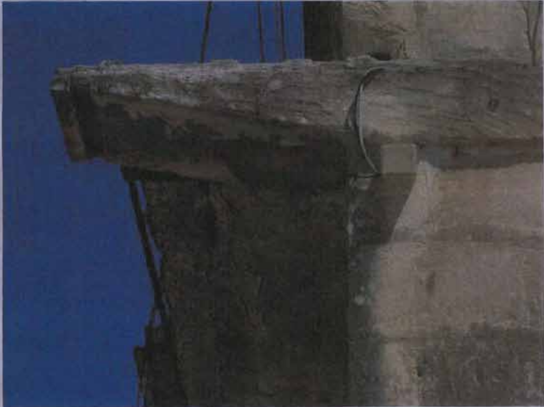
Figure 17: Original sloping stone corbel
